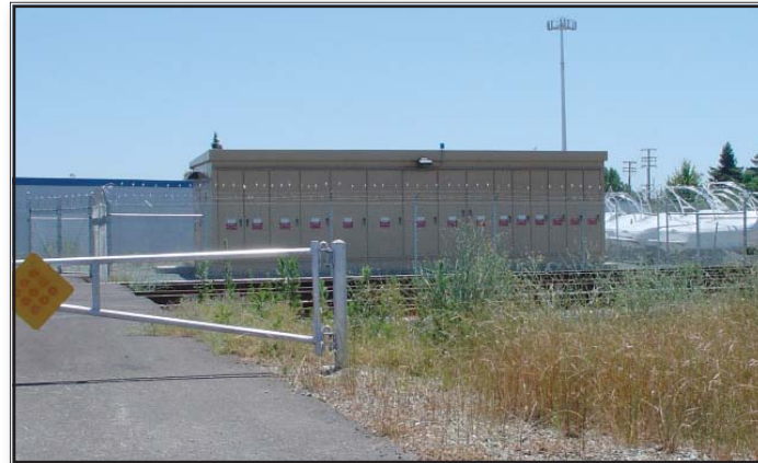
Don't Do This: Equipment exposed to view from roadway and surrounded by razor wire. (Rancho Cordova, California)
