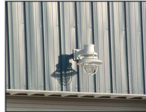
This lighting fixture on the side of an industrial building in Rancho Cordova, California is compatible with the architecture of the building and is shielded
