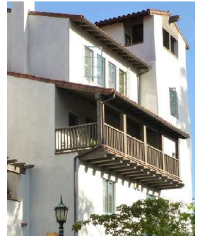
Balcony Overextending Sidewalk
