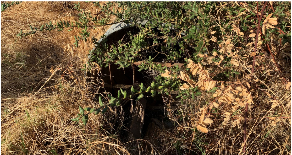
Photo 4 View of culvert at west end of the Area of Interest near fence line shown on Photo 2
