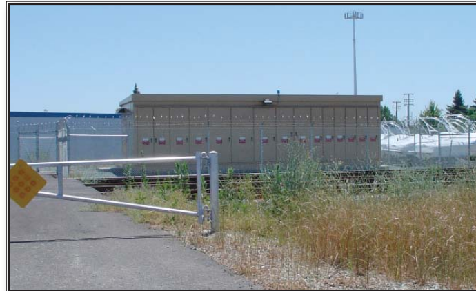
Don't Do This: Equipment exposed to view from roadway and surrounded by razor wire. (Rancho Cordova, California)
