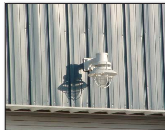
This lighting fixture on the side of an industrial building in Rancho Cordova, California is compatible with the architecture of the building and is shielded
